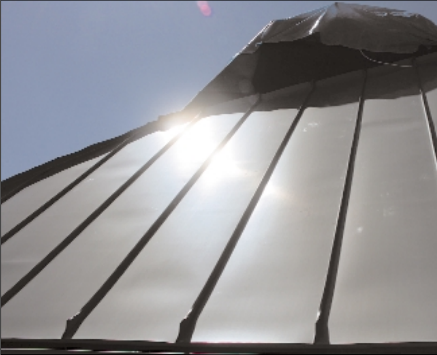
IMAGE: Installing zinc roofing on the Hanson Ecohouse at BRE (Photo: Peter White)
